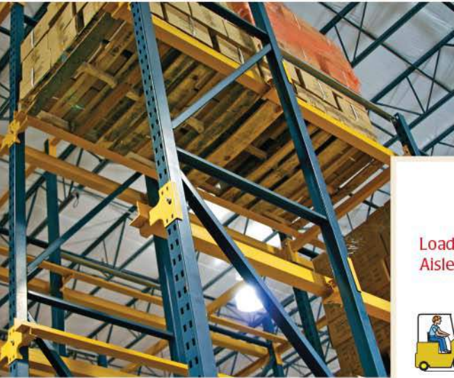
Pallets rest on rails within the bay.
