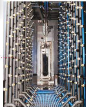
Powder Coat Paint Booth
